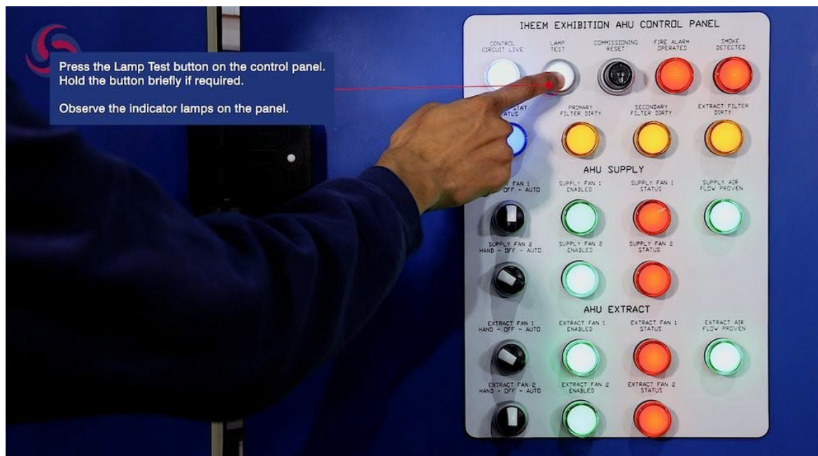
Figure 2. AHU control panel during a lamp test — all indicator lamps illuminate simultaneously, confirming the lamps and their wiring circuits are functioning.
