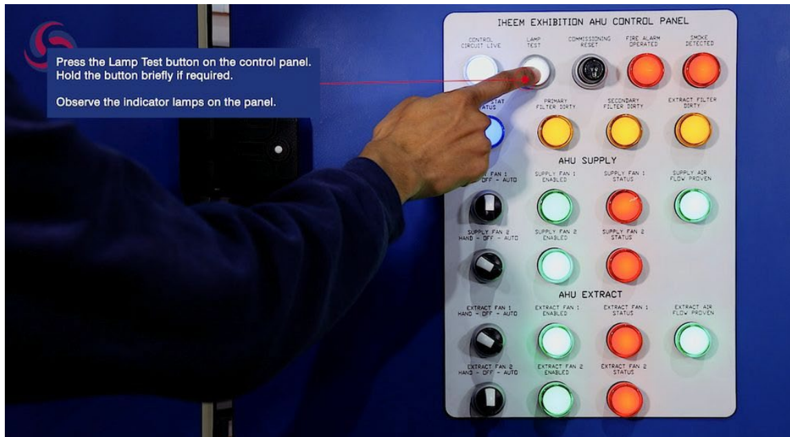
Figure 6. Pressing the Lamp Test button on the control panel and observing the indicator lamps.
