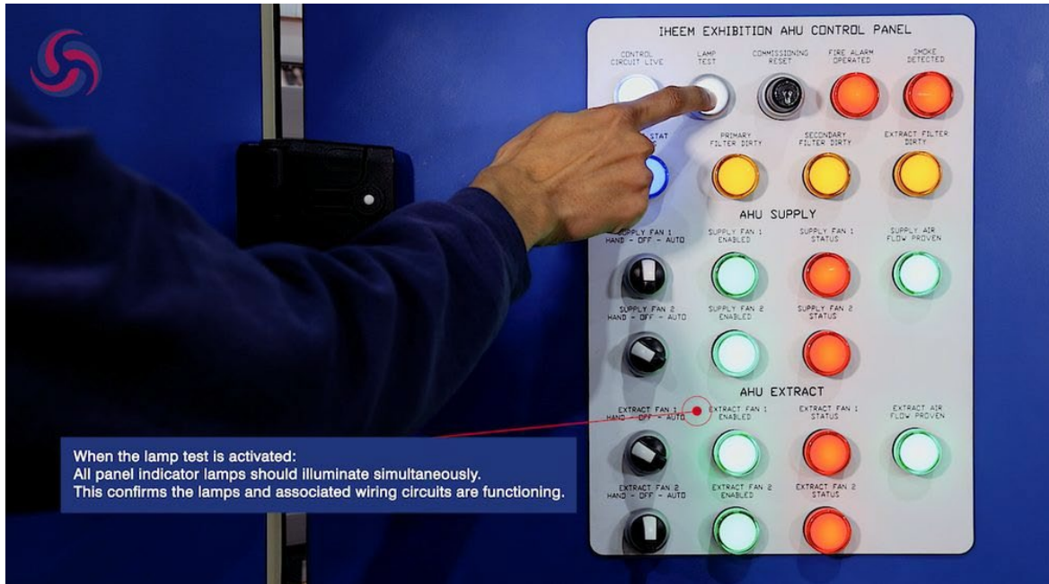
Figure 7. Lamp test active — all indicator lamps illuminated simultaneously, confirming the lamps and wiring circuits are functioning.
