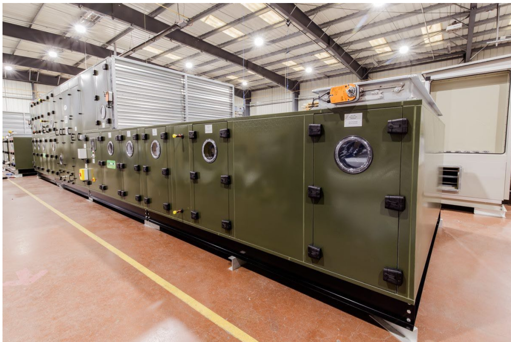
Figure 1. Typical ECE air handling unit.
