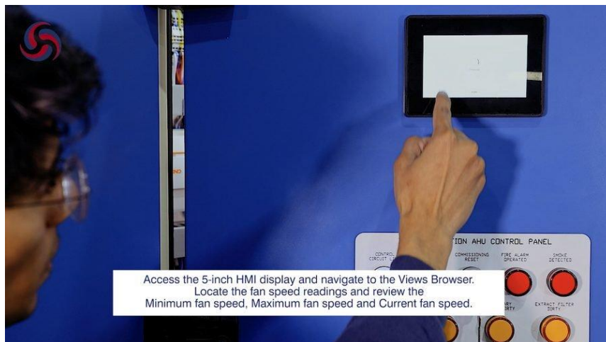
Figure 4. Operating the 5-inch HMI display on the AHU control panel — the starting point for reviewing fan-speed values before a commissioning reset.
