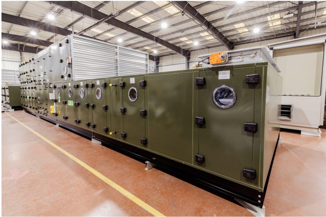
Figure 1. Typical ECE air handling unit with 5-inch HMI display on the AHU control panel.
