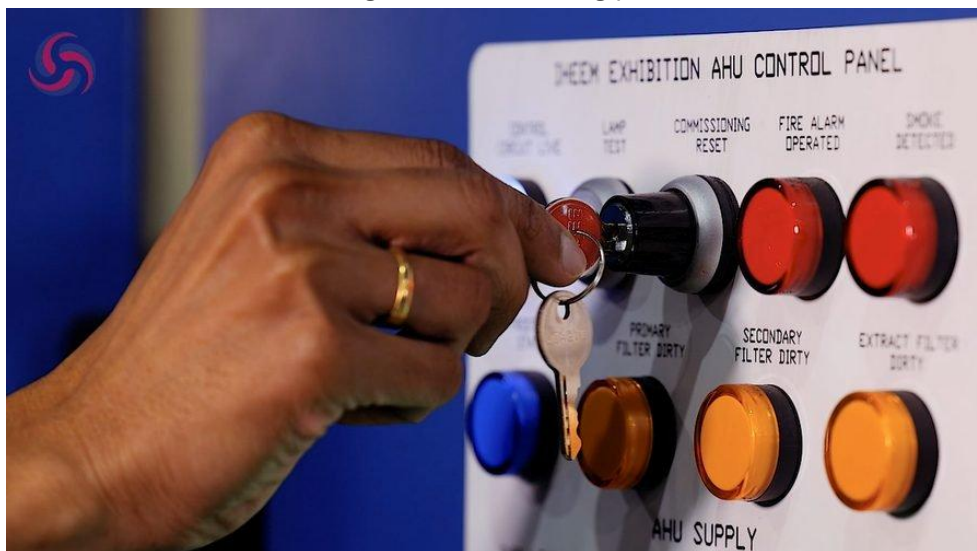
Figure 8. Pressing the Commissioning Reset push-button on the control panel door. Indicator lights confirm the reset function has been activated.
