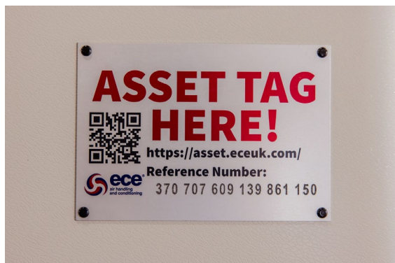
Figure 3. Asset Tag plate carrying the unique 18-digit reference number used to retrieve AHU technical information from the ECE Client Portal.
