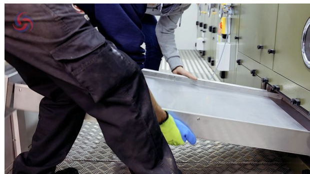
Figure 7. Carrying the removed drain tray clear of the AHU for cleaning and inspection.
