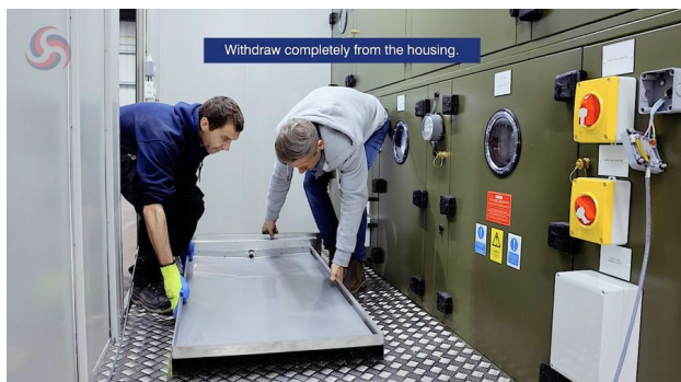
Figure 8. Withdrawing the drain tray completely from the housing — two operatives supporting evenly to maintain tray level.
