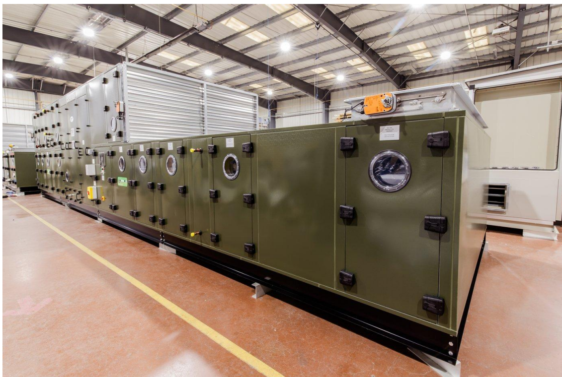
Figure 1. Typical ECE air handling unit. Sensors provide critical feedback to the AHU control system for monitoring and controlling temperature, pressure, differential pressure and airflow conditions.
