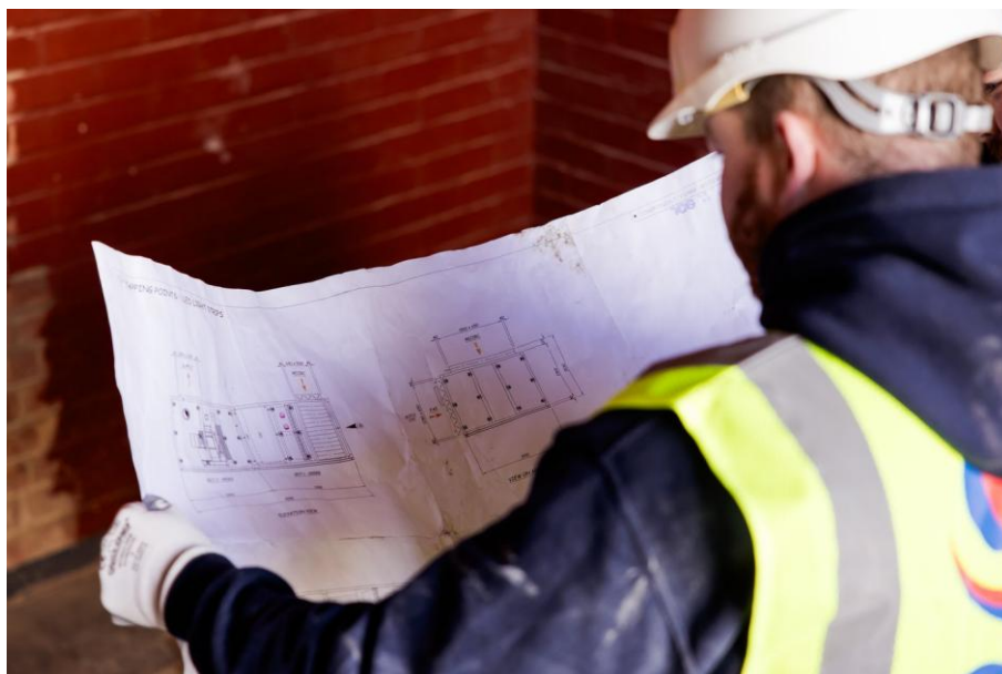
Figure 2. Site personnel in PPE reviewing the certified drawing. Confirm the wiring diagram, terminal numbers and device data sheet before working on any sensor circuit.
