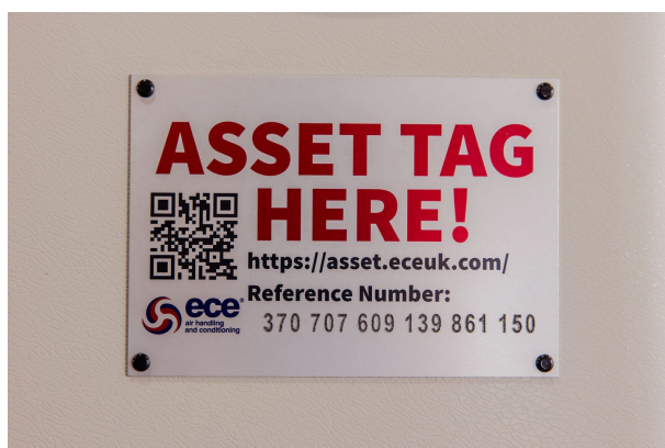
Figure 4. Asset Tag plate carrying the unique 18-digit reference number used to retrieve AHU technical information from the ECE Client Portal.
