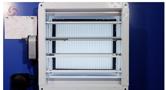
Figure 18. Damper driven fully open by the replacement actuator. Movement should be smooth and unrestricted across the full travel.
