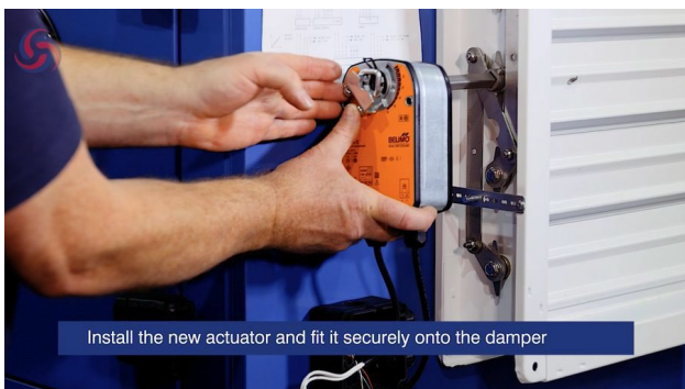
Figure 11. Installing the new actuator onto the damper spindle and aligning it with the mounting bracket.
