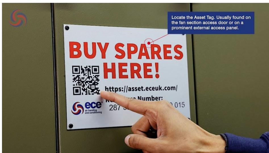
Figure 5. "Buy Spares Here" plate installed on an AHU access door, showing QR code, web address and 18-digit reference number.
