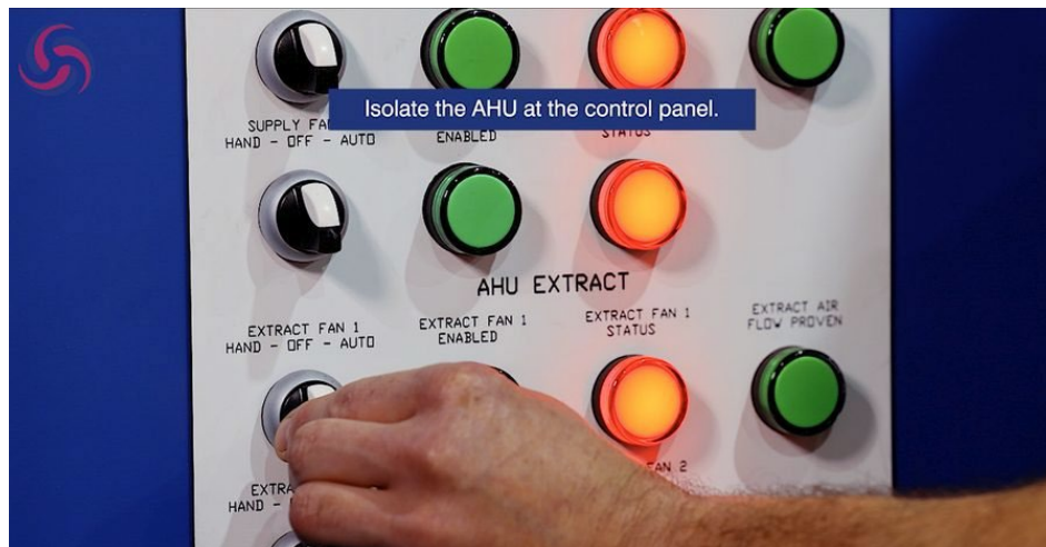
Figure 4. Operative isolating the AHU at the control panel. Confirm the panel is de-energised before proceeding.
