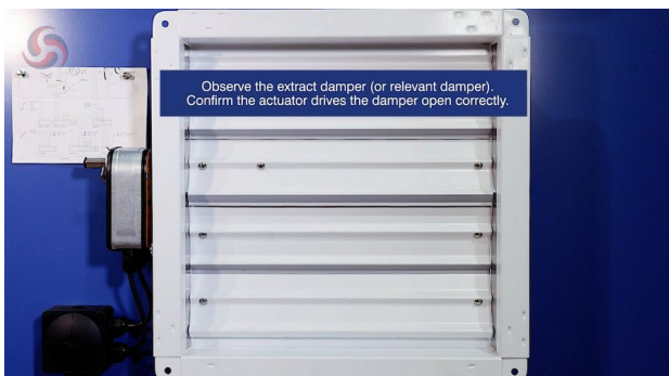
Figure 17. Observing the damper in its closed position before the actuator drives it open.
