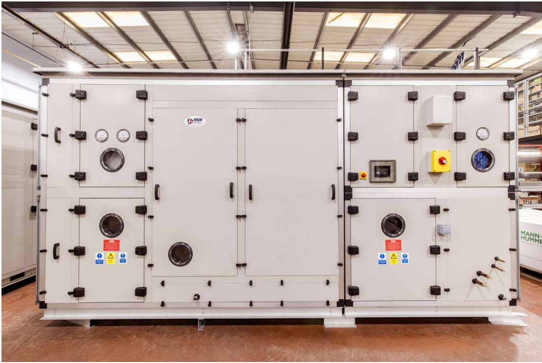
Figure 1. Typical ECE air handling unit showing access doors, control panel and yellow lockable isolator.
