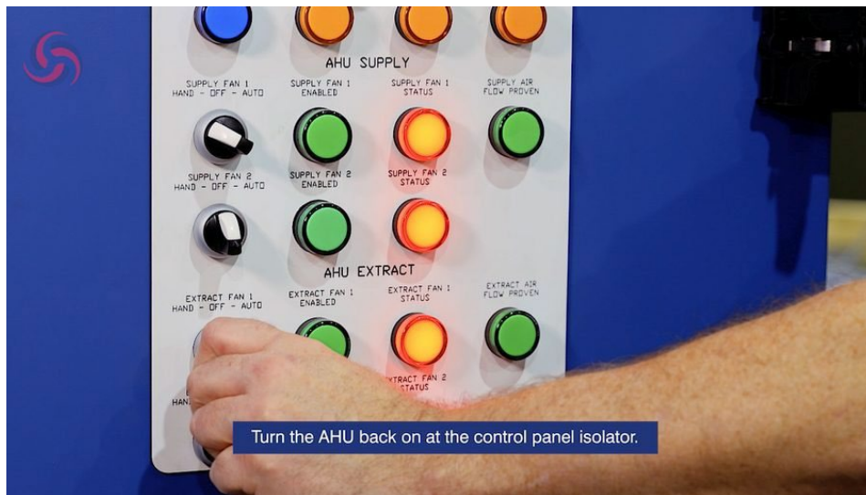
Figure 16. Turning the AHU back on at the control panel isolator. Allow the control system to initialise before checking operation.
