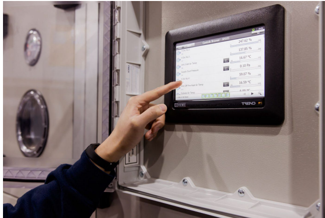
Figure 4. AHU on-board controller used to access Maintenance Mode before opening the filter section.
