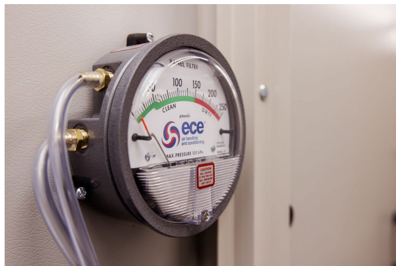
Figure 10. Detail of the Magnehelic gauge showing the two pressure tube connections (high and low) routed to the upstream and downstream tapping points.
