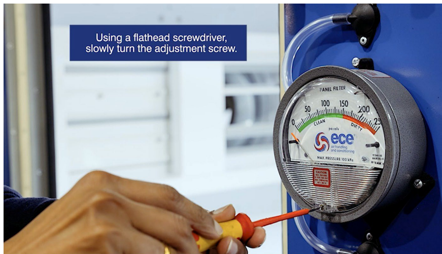
Figure 9. Using a flathead screwdriver to slowly turn the gauge zero-adjustment screw on the front of the Magnehelic gauge.
