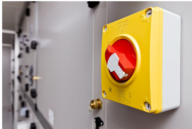
Figure 5. Local fan isolator with red lock-off handle, used to electrically isolate the AHU prior to opening the filter section.
