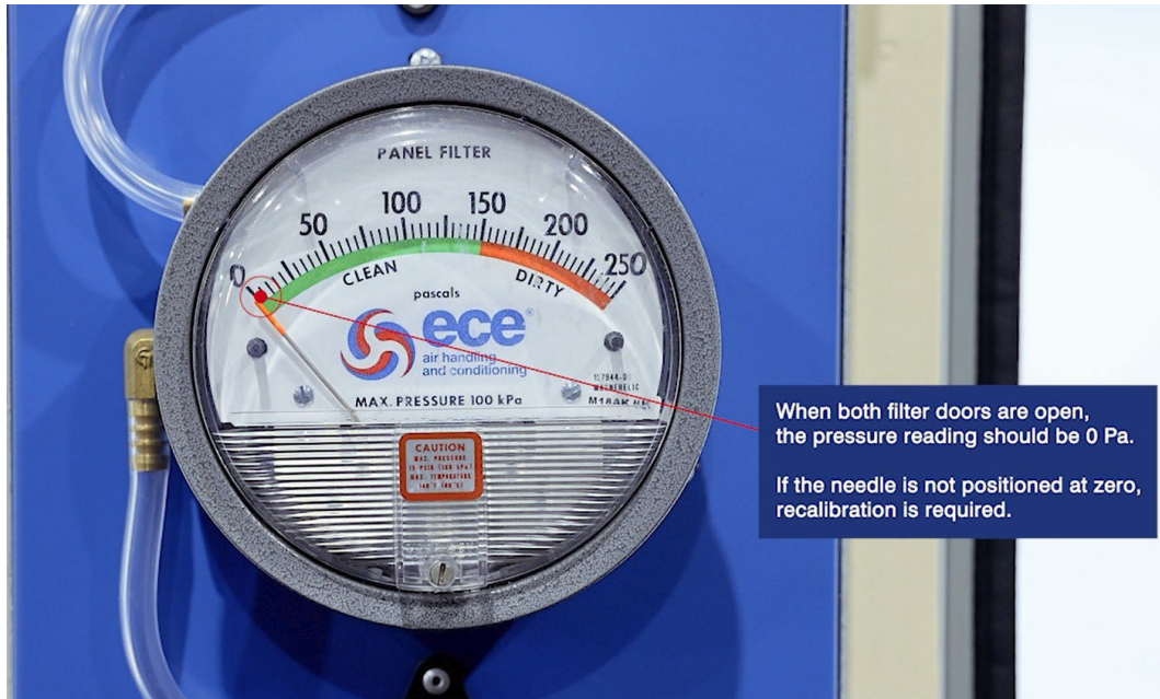
Figure 7. Magnehelic gauge with both filter doors open; pressure reading should be 0 Pa - if the needle is not at zero, recalibration is required.
