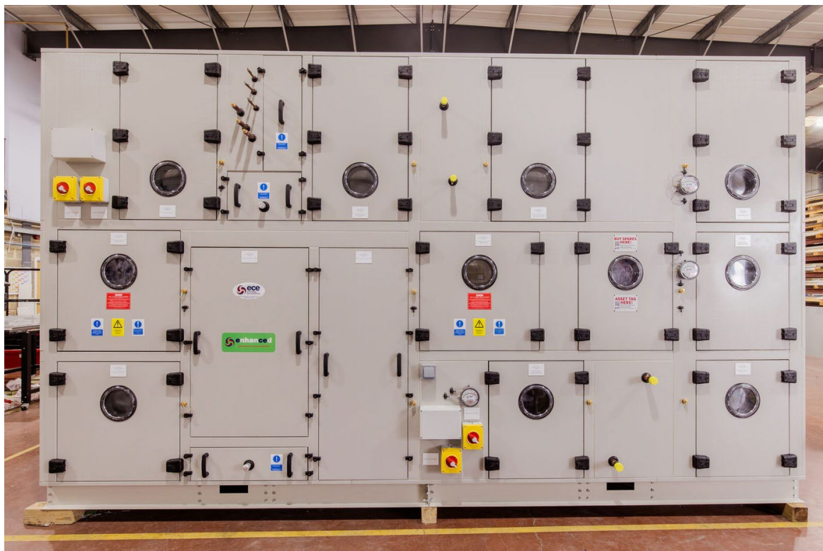
Figure 1. AHU showing multiple Magnehelic differential pressure gauges fitted to monitor filter pressure drop across the unit.
