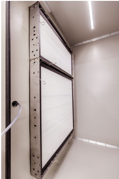
Figure 15. Filter section showing pressure tube tap-off point on the wall adjacent to the installed filter bank.
