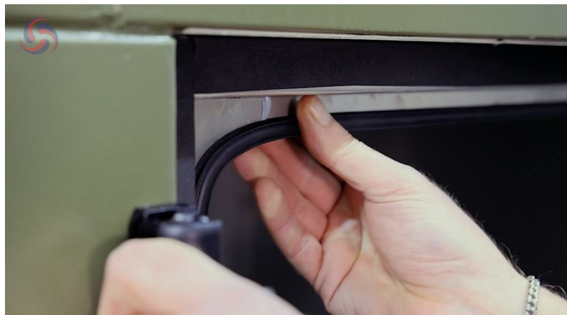
Figure 7. Checking the gasket seal compression around the door perimeter for uniform contact.
