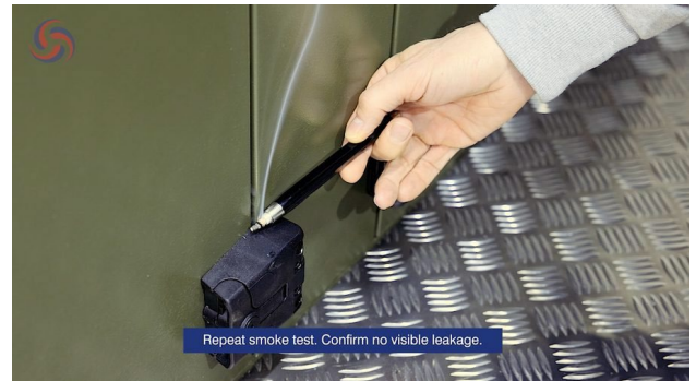
Figure 13. Repeating the smoke test after compression adjustment to confirm no visible leakage remains.
