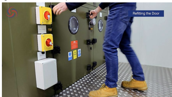
Figure 9. Refitting the door: aligning the hinge barrels and lowering evenly into the hinge seats.
