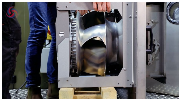
Figure 18. Positioning the replacement fan into the support frame and aligning the mounting holes.
