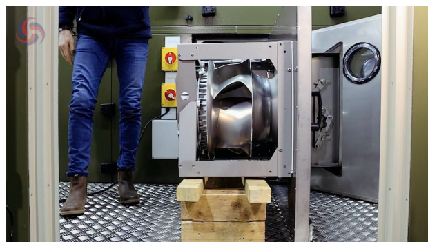
Figure 12. Fan assembly extended fully to the service position. The drag chain supports power and control cabling.
