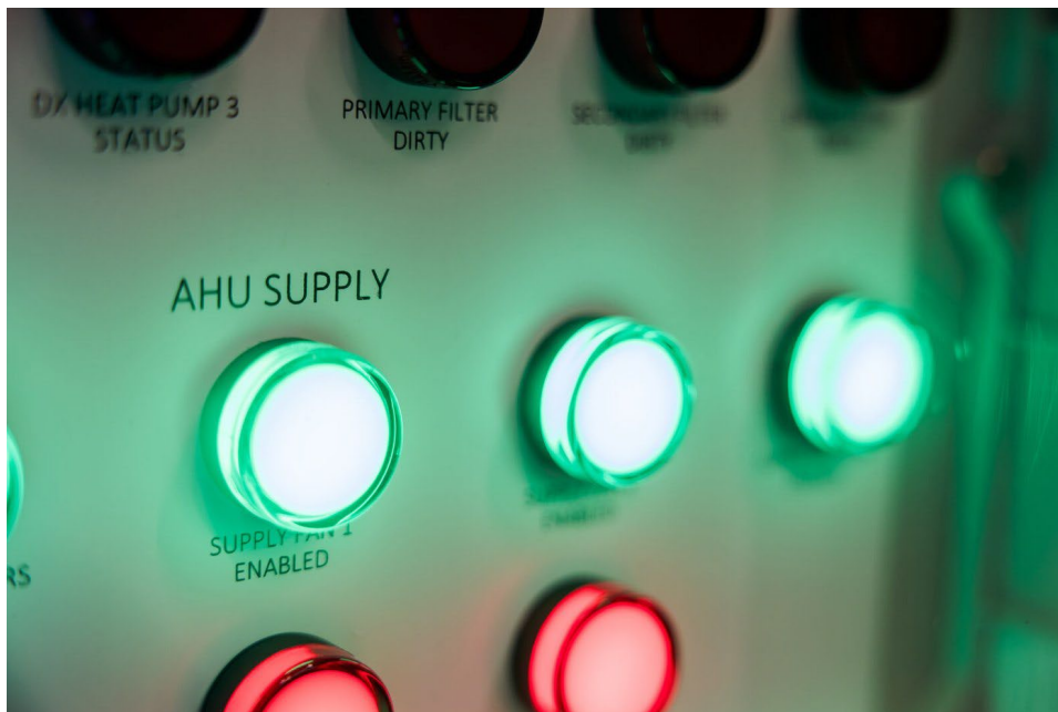
Figure 5. AHU controller status indicators showing fan and AHU operational state.
