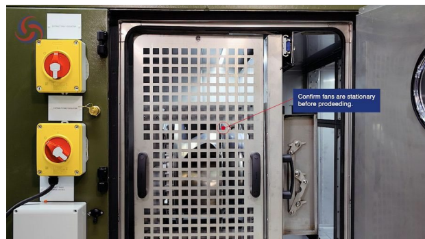
Figure 8. Confirming the fans are stationary before proceeding.
