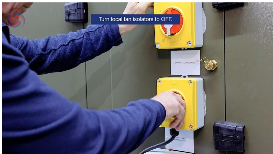
Figure 6. Turning the local fan isolator to OFF before opening the fan compartment. Verify isolation and apply lock-off/tag-out if required.
