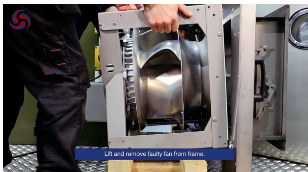
Figure 15. Lifting and removing the faulty fan from the frame. Observe safe manual handling practices.
