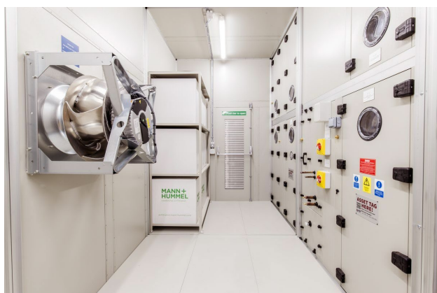
Figure 16. Spare EC plug fan stored on the wall-mounted storage bracket inside the plant room.
