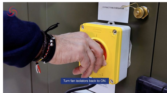
Figure 24. Turning the fan isolators back to ON and exiting maintenance mode to restore normal duty.
