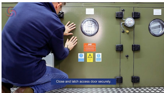
Figure 23. Closing and latching the access door securely once the fan assembly is fully secured.
