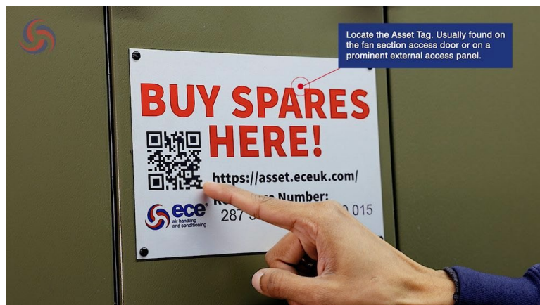
Figure 3. “Buy Spares Here” plate installed on an AHU access door, showing QR code, web address and 18-digit reference number.
