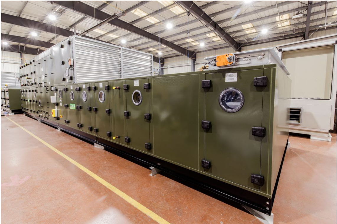
Figure 1. Typical ECE air handling unit. Every ECE AHU is fitted with a unique "Buy Spares Here" QR plate giving direct on-site access to site-specific parts and spares via the ECE Client Portal.
